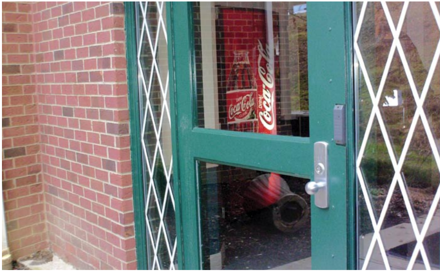
▲ Exterior of dormitory door with EL exit device shows proximity card reader that activates the electric latch retraction function.
